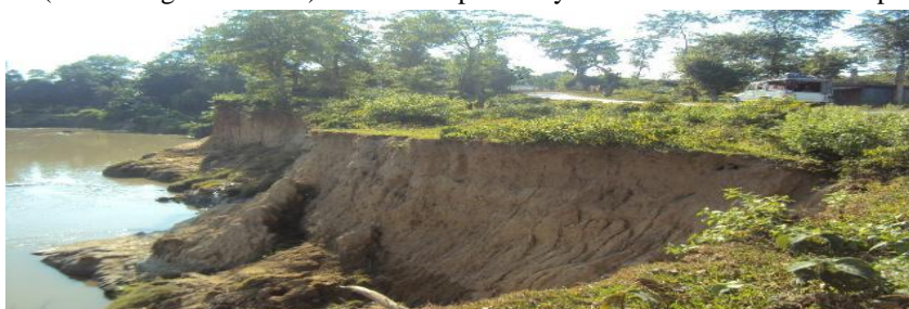
Fig 10: Teliamura-Khowai State Highway occupied by the River Khowai at Purba Kalyanpur.
